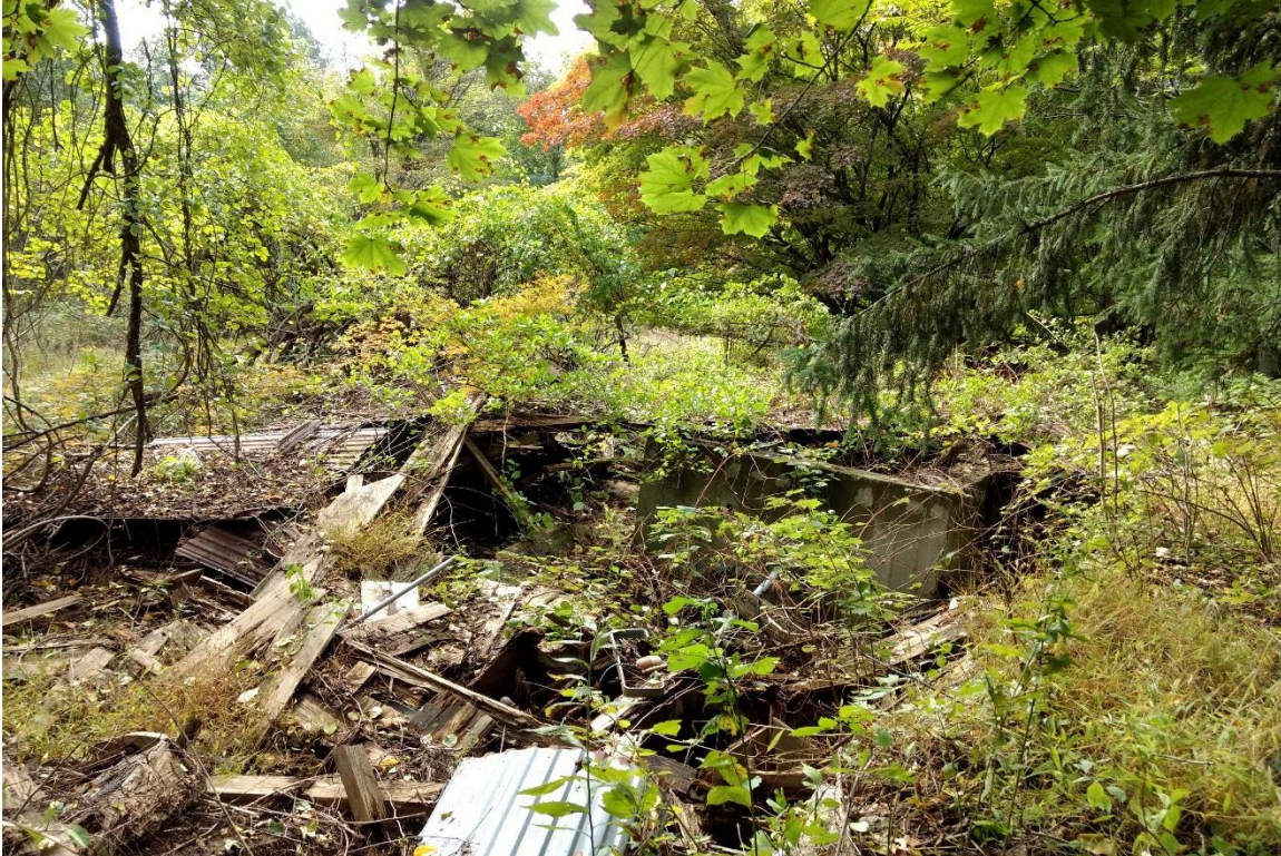
Photo 12: A collapsed structure holding pool house equipment is located on the western side of the barn overlooking the pool. View to the west.
