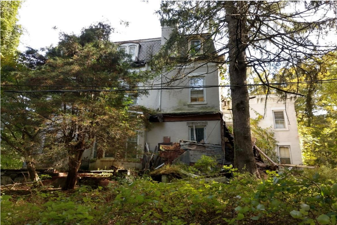
Photo 18: The porches around the exterior of the structure have collapsed. View to the east.
