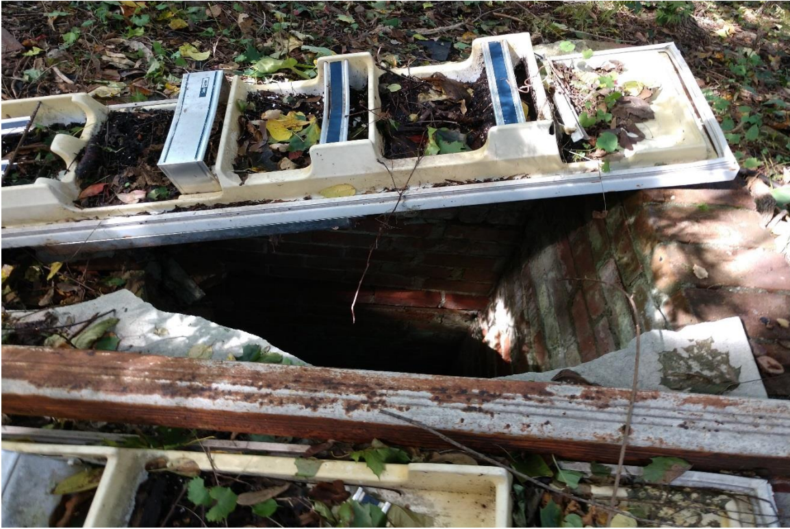
Photo 20: A brick dry well is located to the southwest of the former hotel. View to the west.
