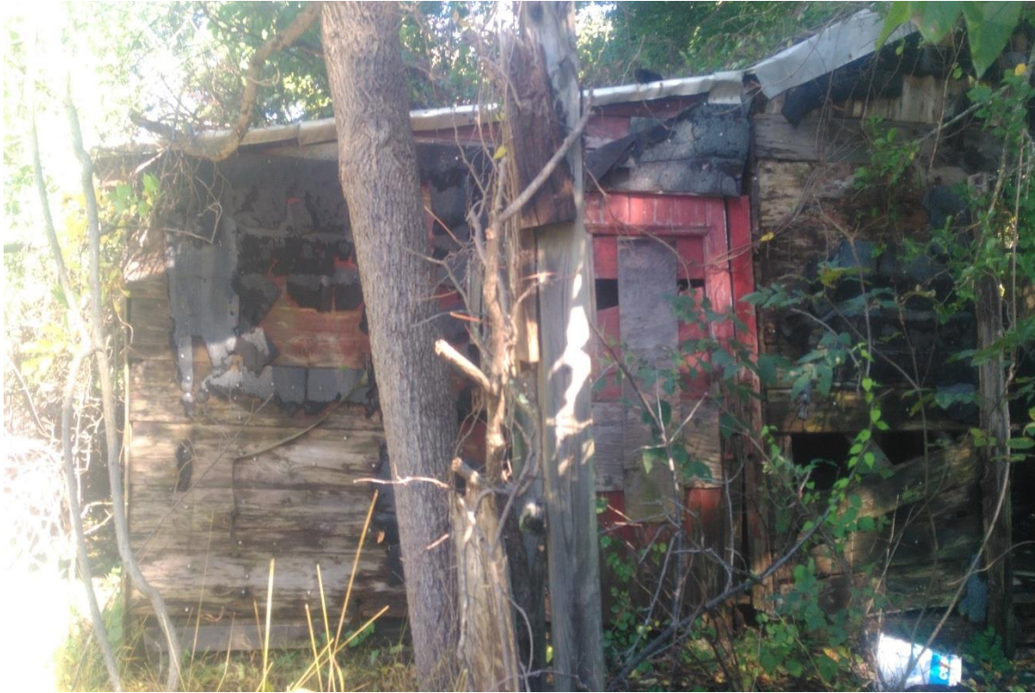
Photo 13: A small livestock shed or cabin is located in the western portion of the parcel. The current caretaker reports that these structures were used in the past by Girl Scouts.
