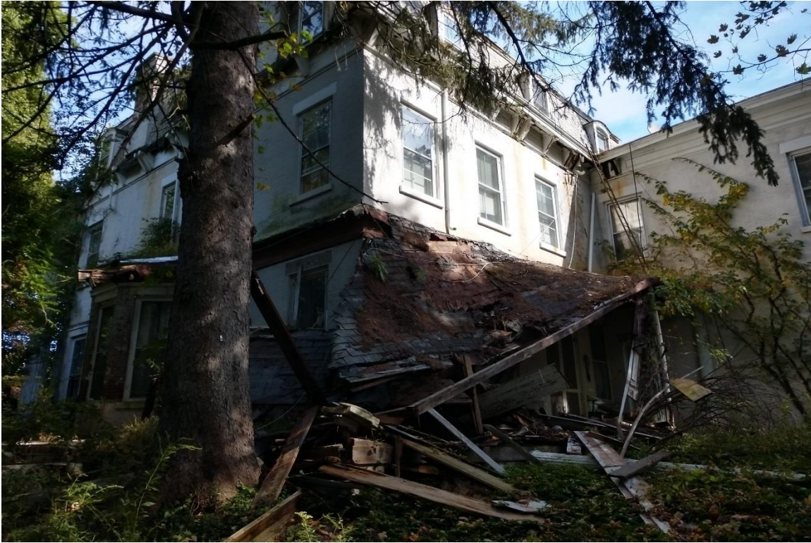
Photo 9: The porch on the southwestern side of the former hotel has collapsed, and debris surrounds the base of the foundation. View to the northeast.
