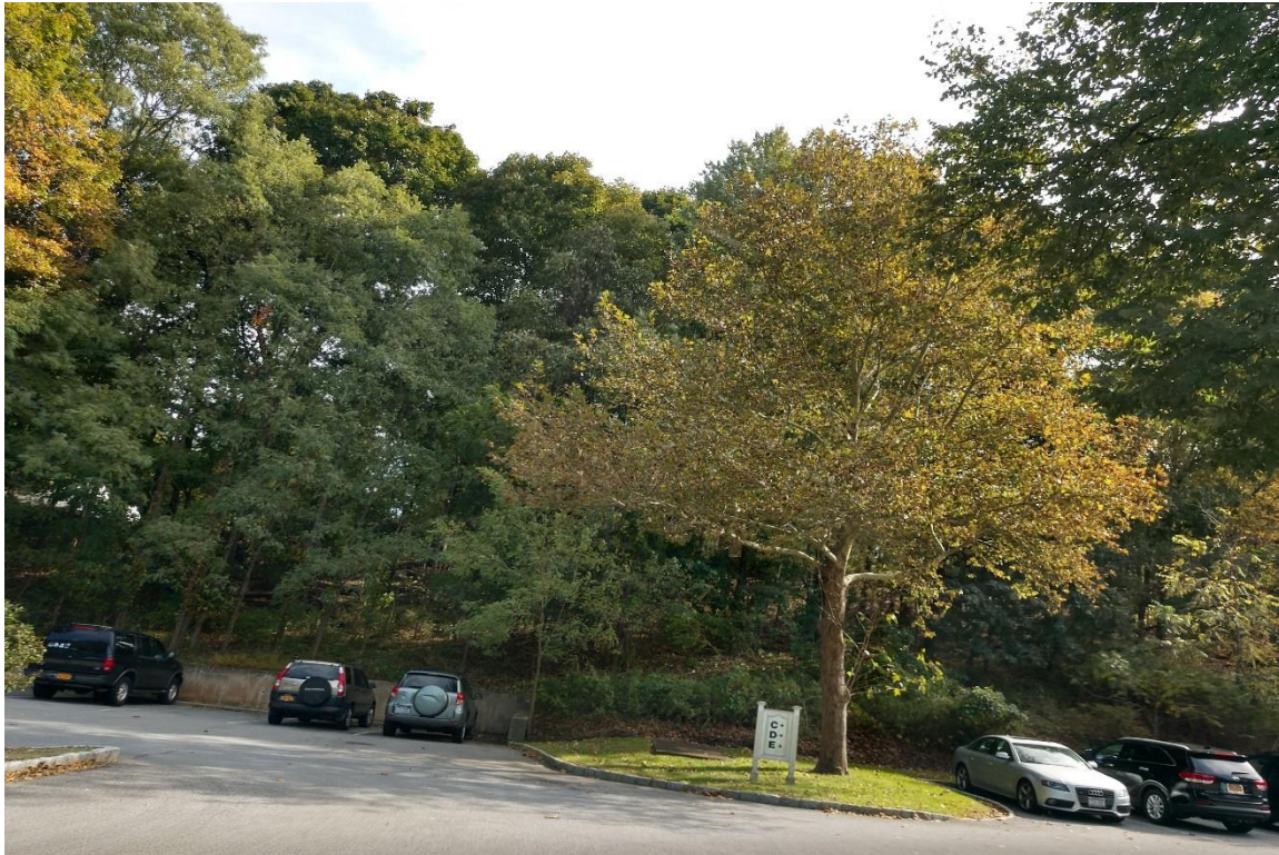
Photo 2: The parking lot is bordered to the east by steep slopes and a concrete retaining wall. View to the east.
