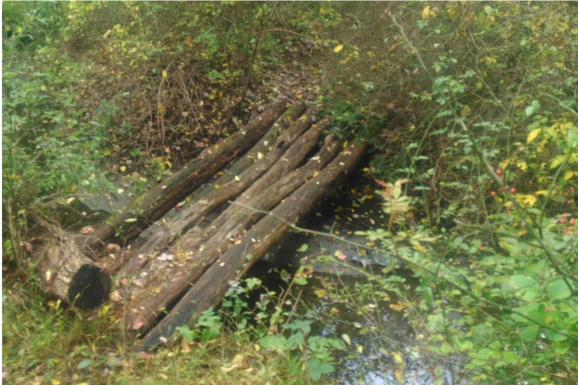
Photo 14: A wooden makeshift bridge crosses the small stream in the southwestern portion of the Project Area. View to the west.
